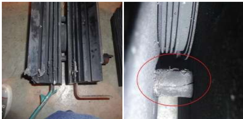
Figure 3. Damage to the Thyristor in the Excitation System
